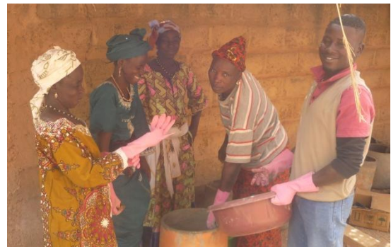
Figure 5: Women are learning how to apply the cement layer during a workshop.
